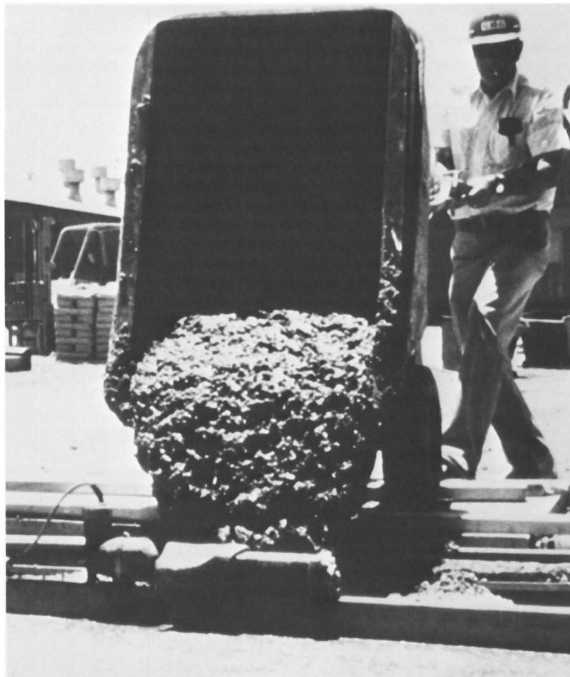
Figure 5. Transporting and pouring the hot sulfur concrete with an insulated motorized concrete buggy.
